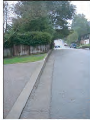
Fencing encroaching on right-of-way
