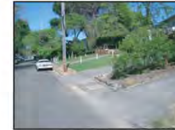
Driveways do not meet ADA slope
