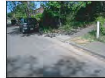
Existing sidewalk is incomplete
